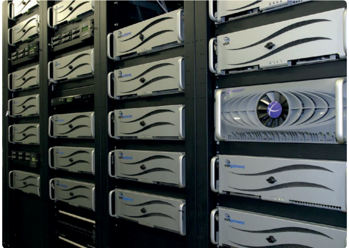
Four VSN storage racks and fully redundant network system
