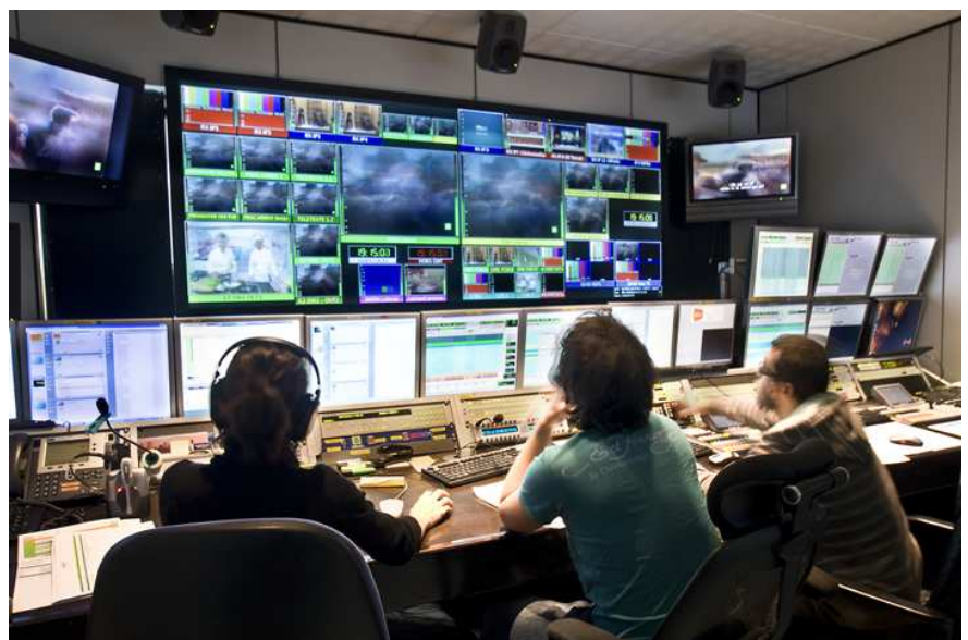
Master Control Room in laSexta
